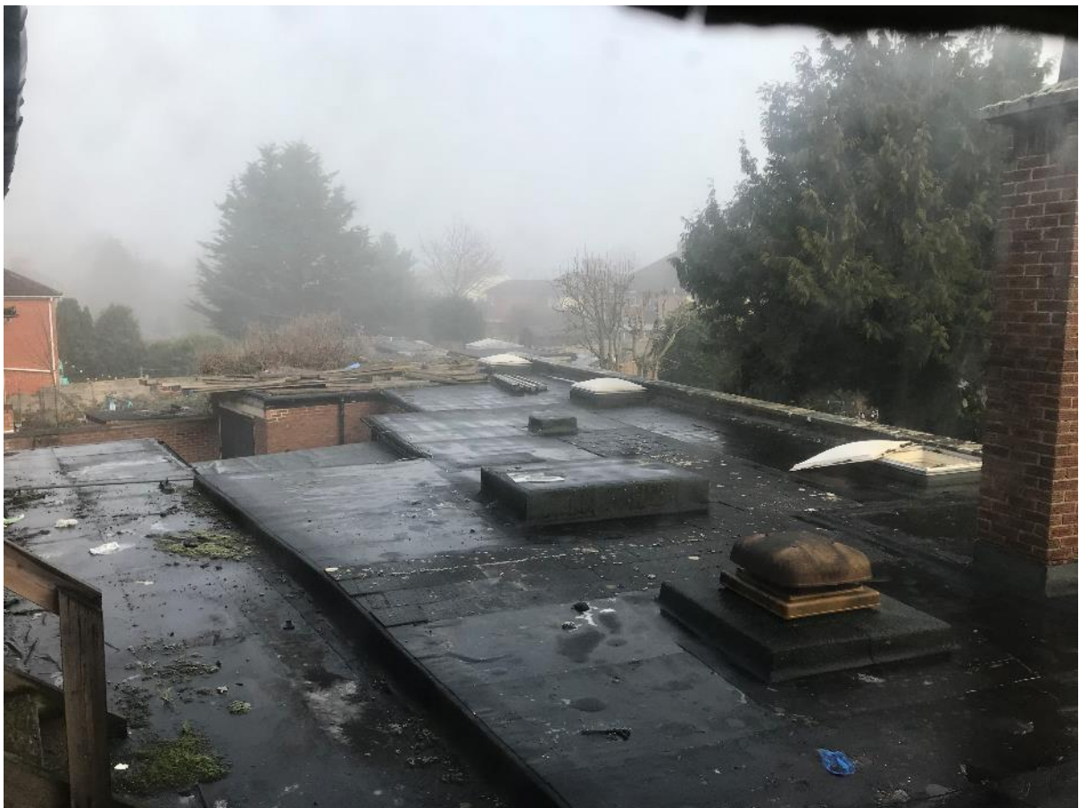
Poor condition flat roofs
