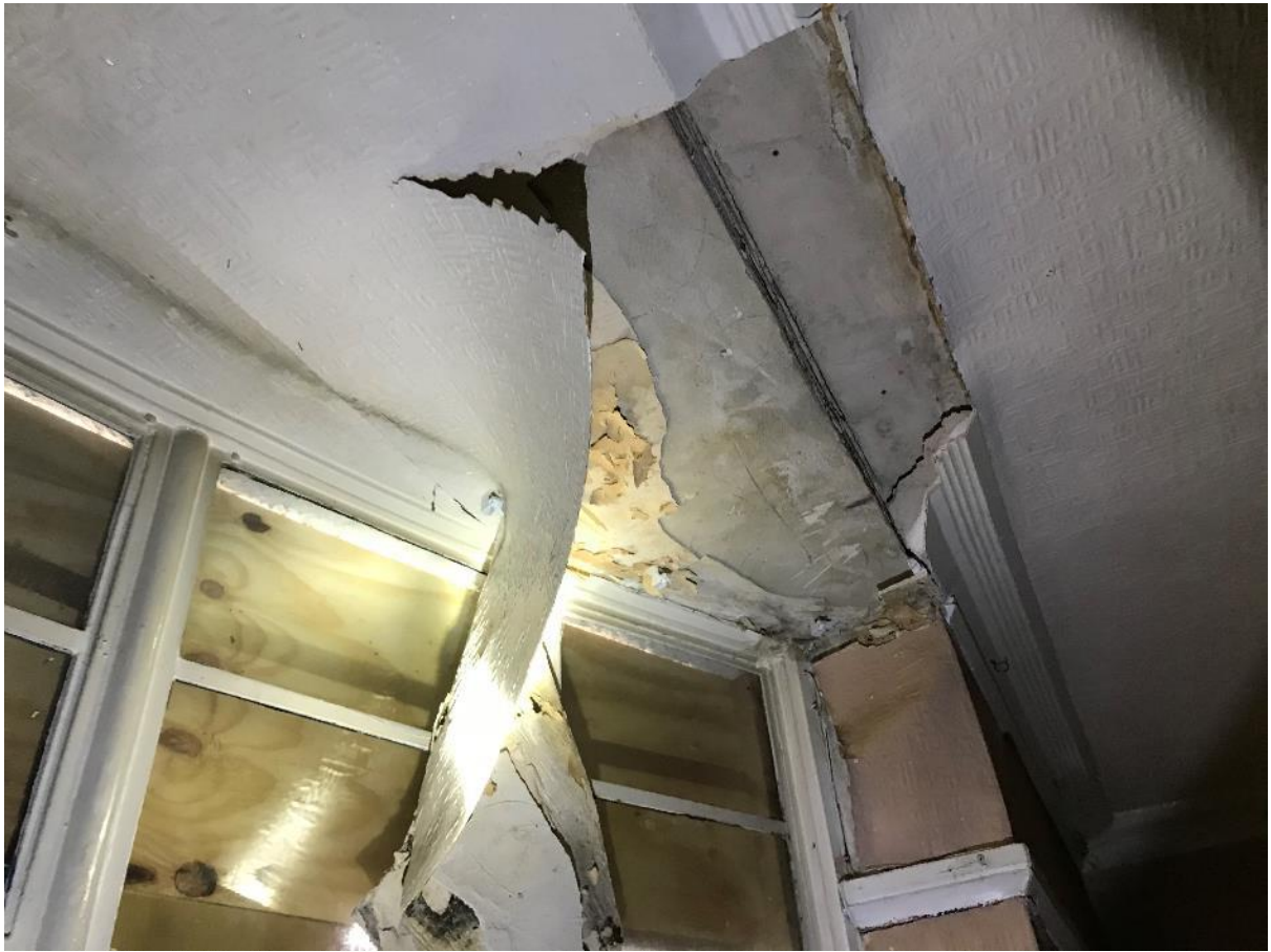
Roof leak / collapsing ceilings
